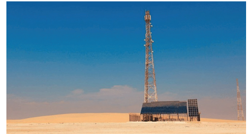
Telecom tower with solar and battery
